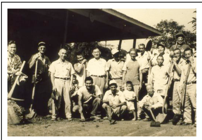
1962 – 1964 Some of our “true-working” pioneers, happy that the temple’s metal framing and roof are up.
